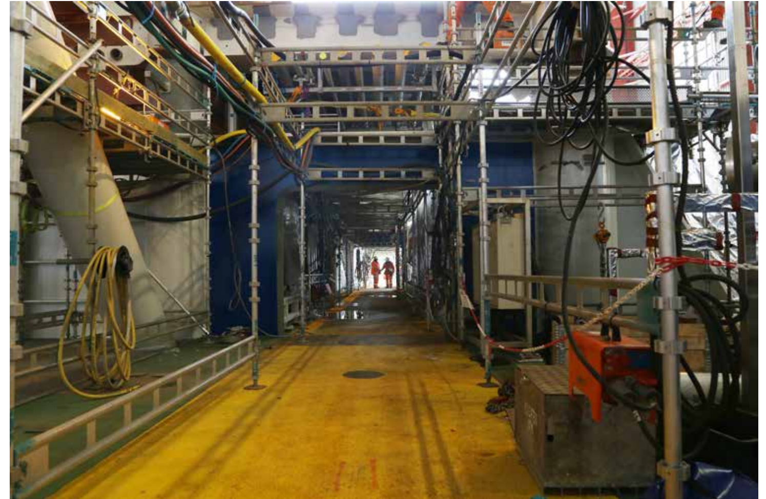
Outfitting. The topsides for the Johan Sverdrup quarters platform is starting to look like an offshore installation.
